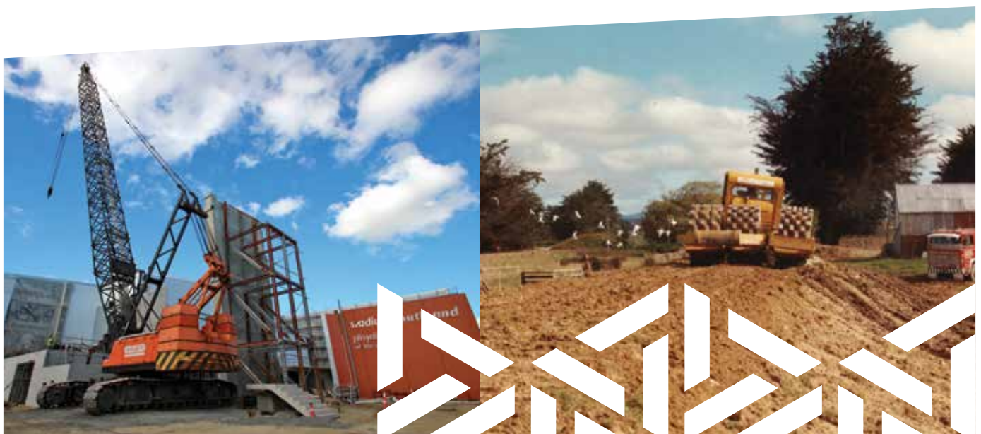
Right: Repair work being undertaken to the stopbanks of the Mataura River by the Tannery corner following the floods of 1987
