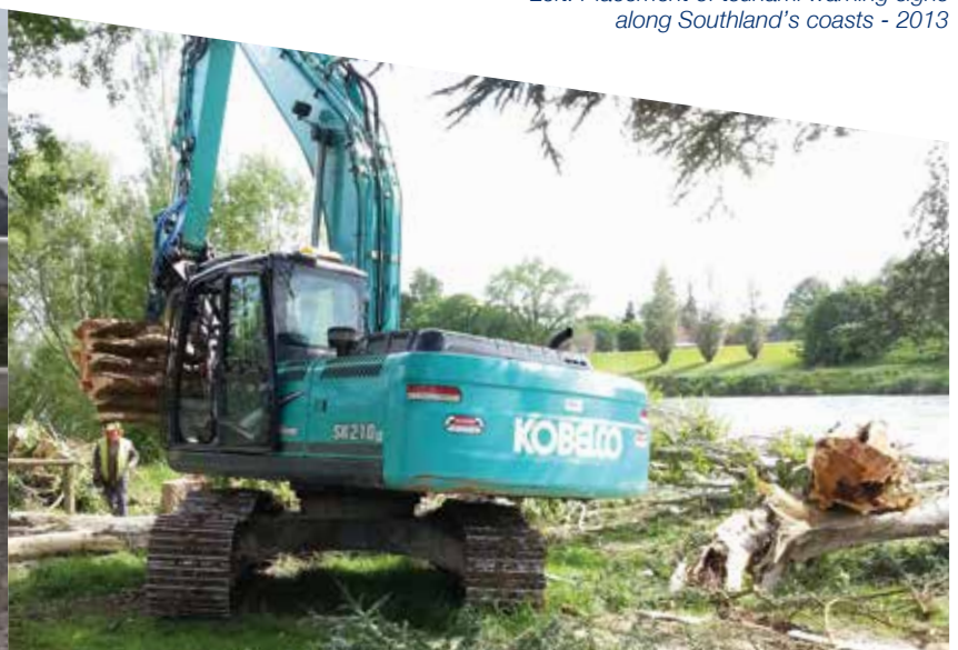
Right: Removing willows from the Gore Floodway to allow the Mataura River to flow unhindered in this area.
